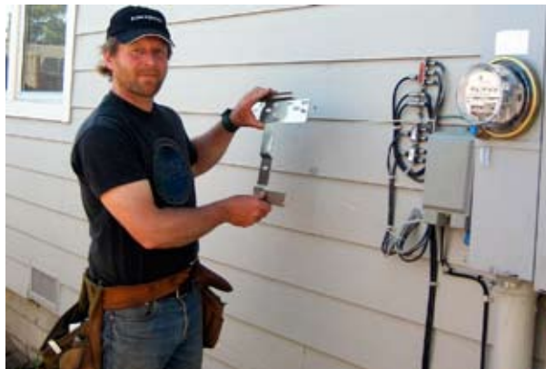
Bruce Erickson, owner MSS setting an inverter HFH GOES SOLAR by Bruce Erickson
